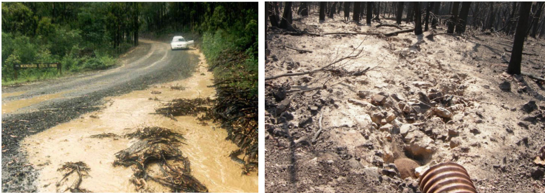
Figure 4. Examples of road-related erosion. (left: Photo Gary Sheridan) Road runoff and detachment of sediment from the road surface. (right) Hillslope erosion caused by discharge from the road surface after a bushfire.
