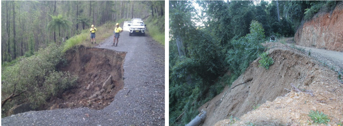
Figure 6. (left) Example of a road constructed in the 1950s using side-casting techniques (where excavated material is simply pushed over the edge of the roadway), and has collapsed during a large precipitation event in 2013 (Photo FCNSW). (right) Failure in road batter located in a very steep hillslope in response to east coast low heavy precipitation event (441 mm in 3 days)
