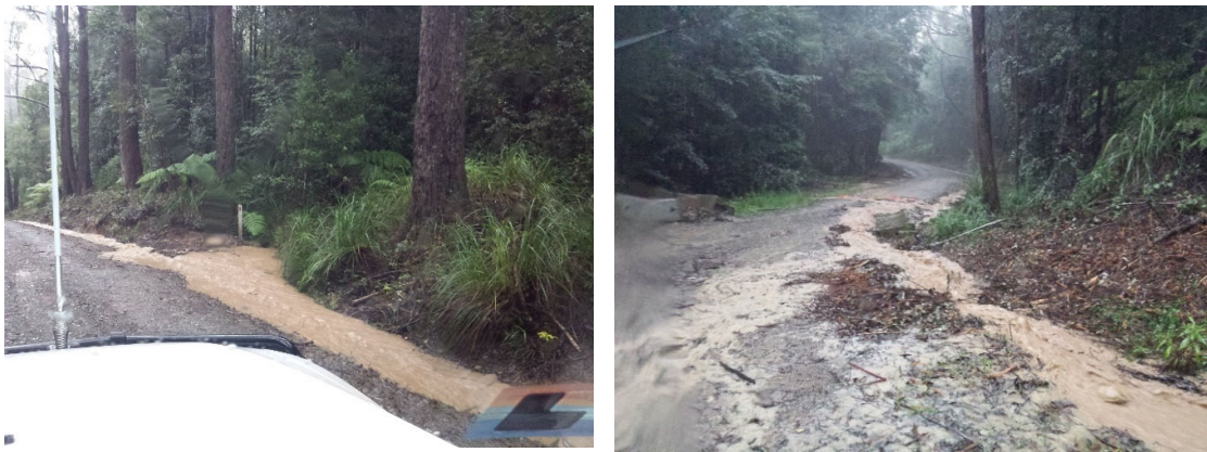
Figure 5. Examples of road-related erosion. (left: Photo Ross Peacock) Road runoff overwhelms culverts (left) and transports sediment and debris downslope (right: Photo Ross Peacock)
